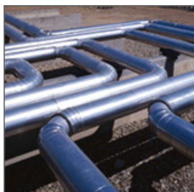
Hydrogen delivery via pipeline
